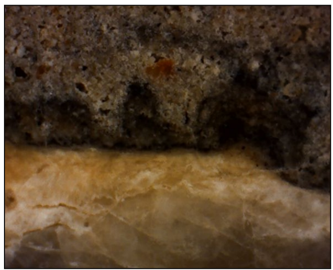
Fig. 22: Interface between the black crust and the substrate in sample B1 (magnification 200×).
