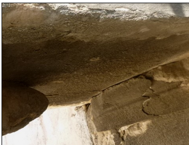
Fig. 7: Deterioration patterns in sampling area of sample B1 (Ephorate of Antiquities of Athens).
