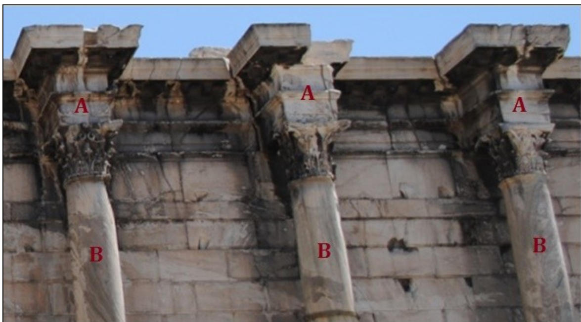
Fig. 4: Western façade with areas built in Pentelic marble (A) and Karystos marble (B) (Personal archive).
