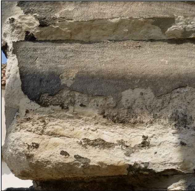
Fig. 9: Deterioration patterns in sampling area of sample B2 (Ephorate of Antiquities of Athens).
