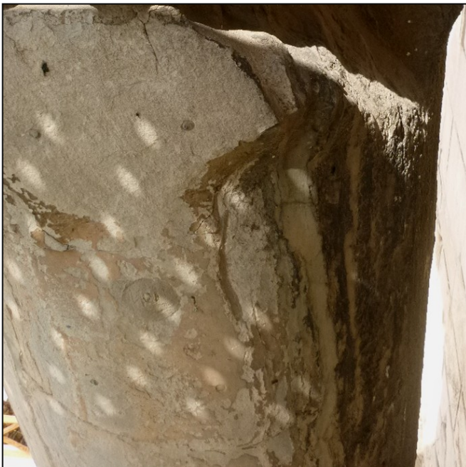
Fig. 13: Deterioration patterns in sampling area of sample B4 (Ephorate of Antiquities of Athens).
