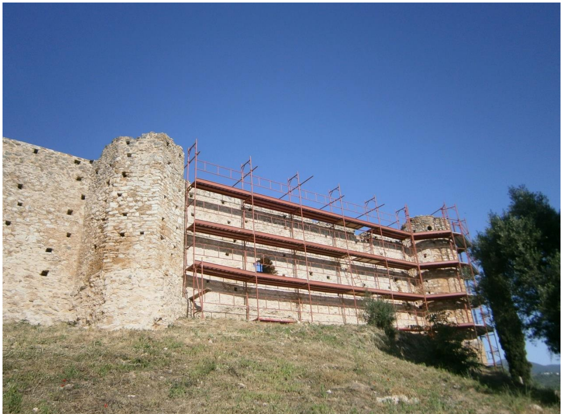
Photo 14: Restoration works at the castle during 2013-2015 (archive of the Ephorate of Antiquities of Messenia)
