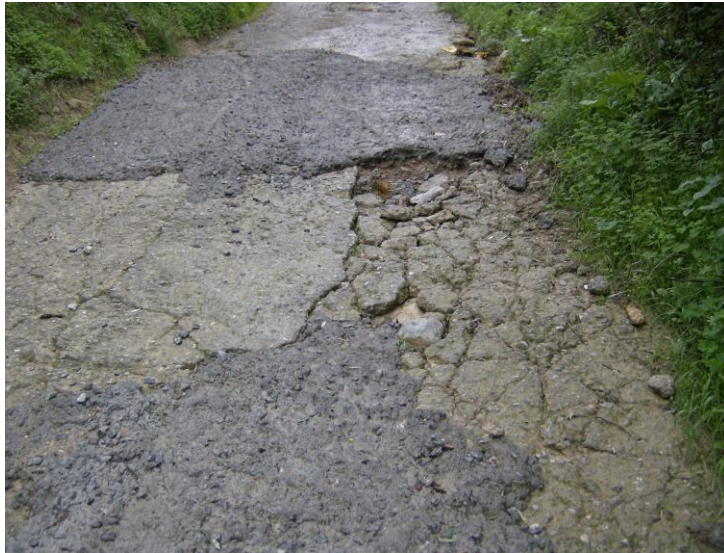
Figure 23. The cemented road full of puddles (photo by S. Kalogeropoulou)
