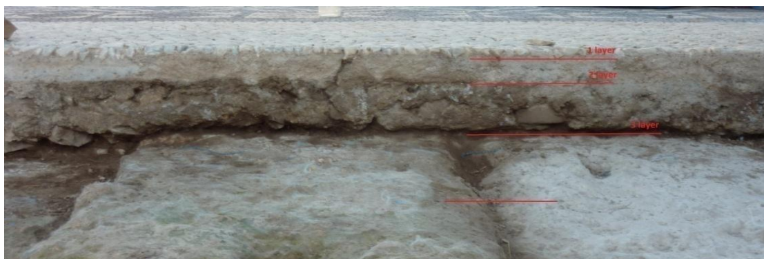
Figure 18. East side of mosaic floor A. In figure: Red line (a) area. Mosaic substrate mortar layers on top of big ashlars. (Mantzana E.)
