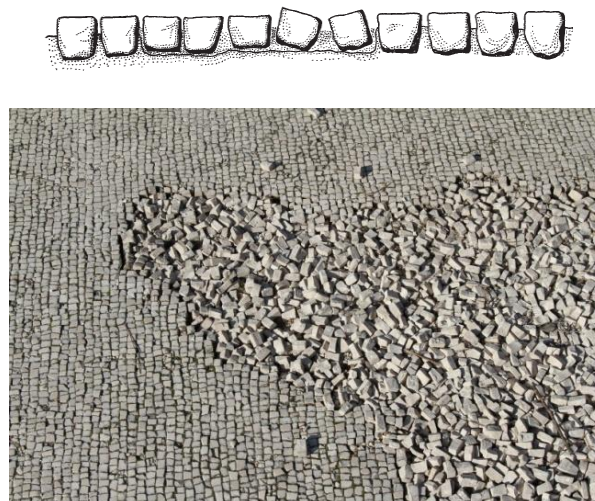
Figure 31. Detached tesserae in mosaic floor in Ostia of Italy. (The Getty Conservation Institute 2003 ( www.blog.travelmarx.com/2010/11/mosaic-and-marble-floors-of-ostia.html ))
