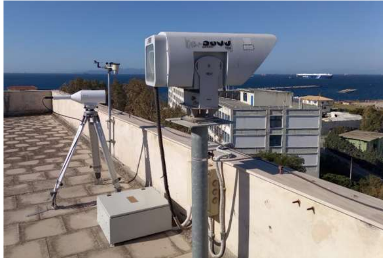
Figure 7.16. The MRV TS5000/155 FSO system, co-located with the BLS450 scintillometer and the ambient weather WS-2000, weather station on the roof of the laboratory building of the Hellenic Naval Academy.
