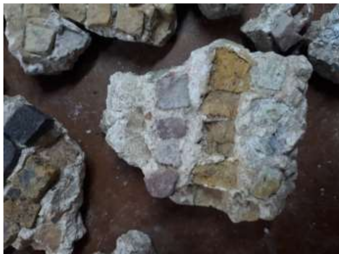
Figure 25: Wall mosaic fragment conserved in 2012, now powdering and deteriorating. Photo taken by Paige Van Tassel.
